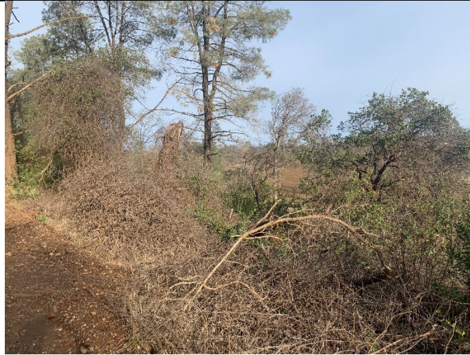
Before: Typical conditions on Jerusalem Grade Road prior to mastication in Middletown, CA.
