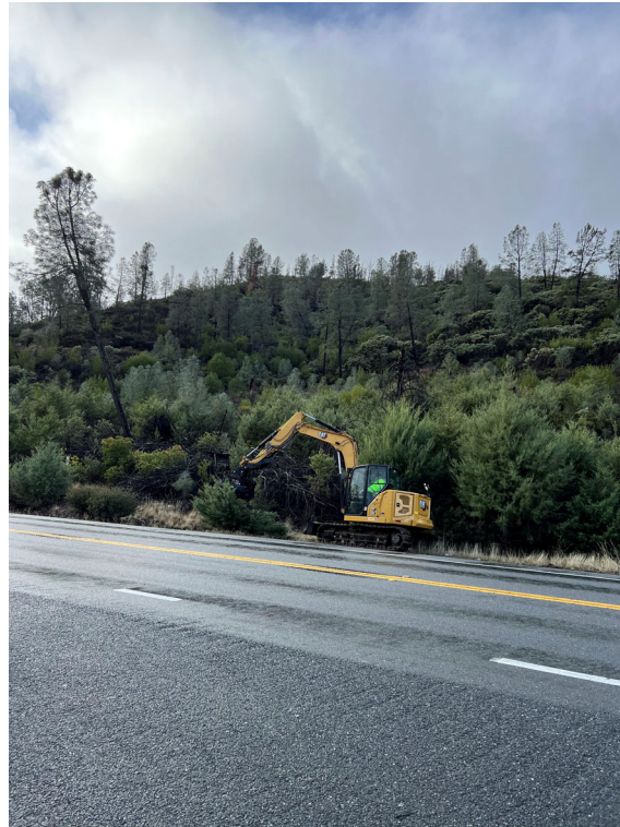
Before: SLFPD excavator masticator beginning work along Hwy 29 south of Middletown, CA.
